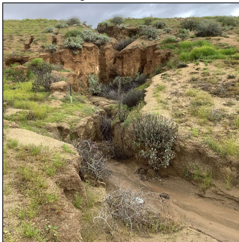
Photo 4: Facing north, close up of eroded area and exposure.
