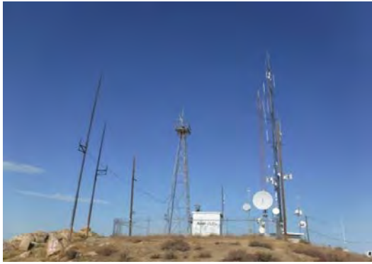
Box Springs Communications Site
