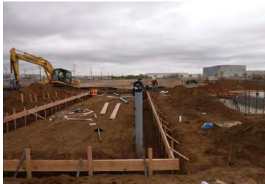
Kitching Substation and SCE Switchyard / Facility Upgrades
