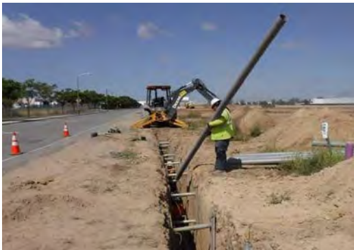
Kitching Substation Feeder Line - Modular 12kV
