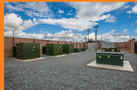
Moreno Valley Utility South Industrial Substation
